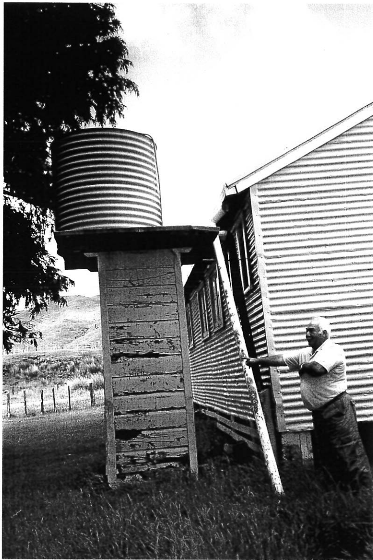
Trustee Russell showing the water tank stand which needs rebuilding
