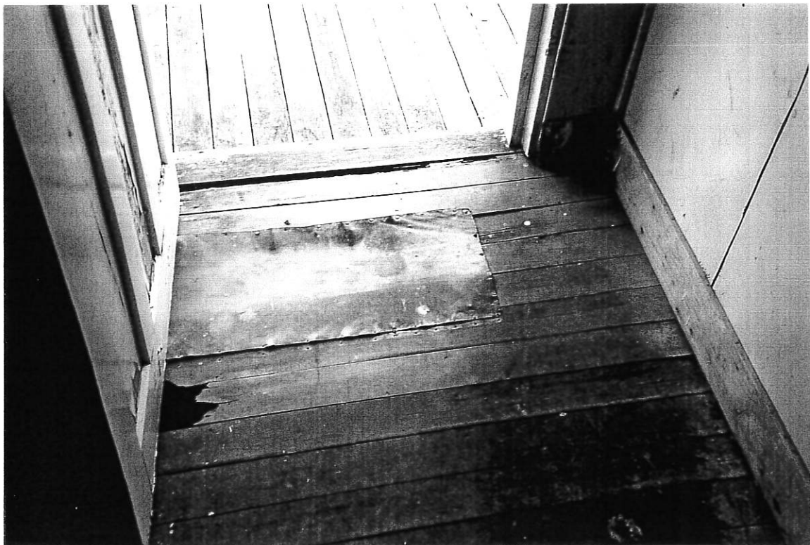
is part of the Shearer Quarters floor needs replacing EGH 12/04
