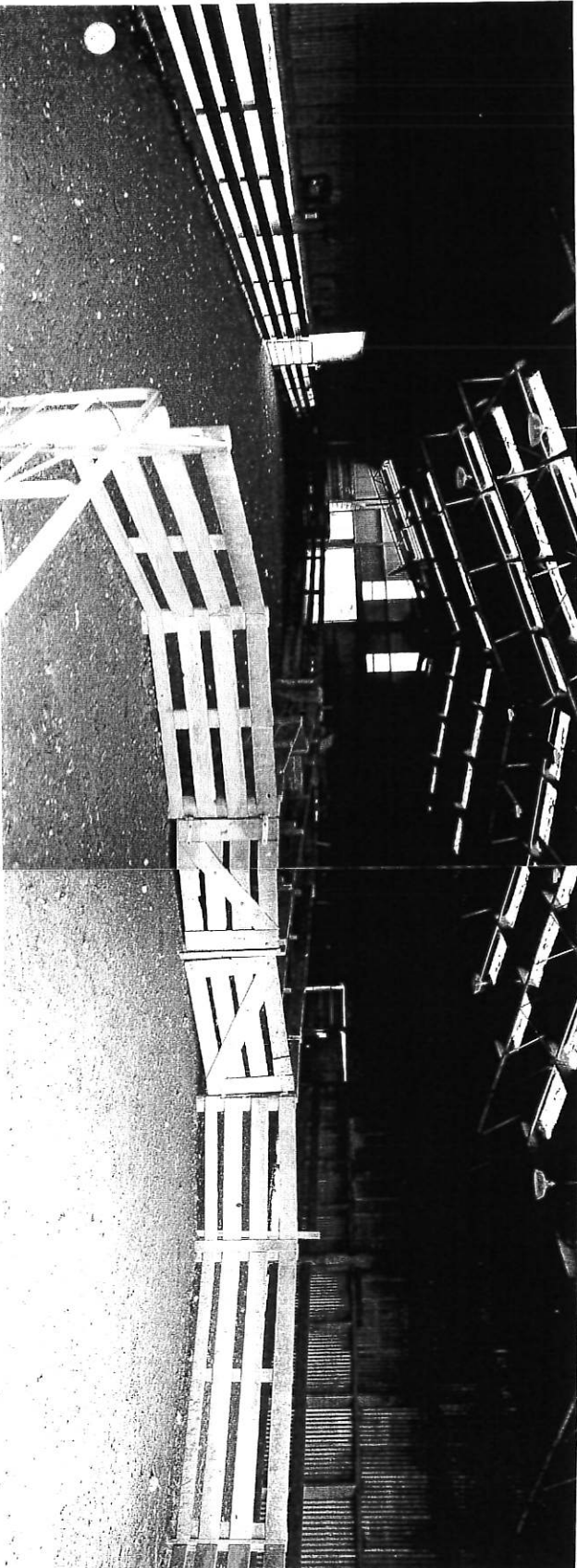
The weathered although very old is sound, well painted and maintained. Covered yards are at right.
